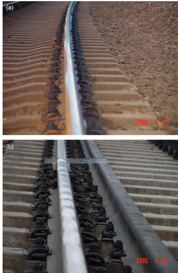
Fig. 2. (a) Long pitch corrugation on low curved rail at 120 km/h and (b) medium pitch corrugation on high curved rail at 80 km/h.
